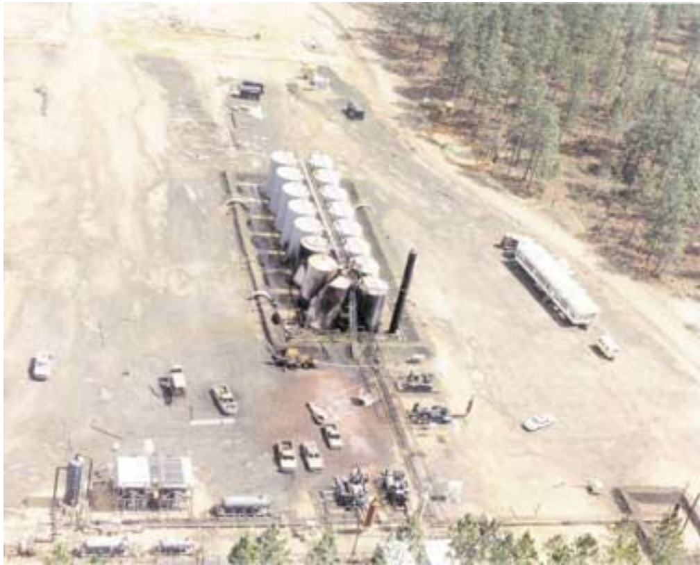
Figure 1. Aerial View of the Temple 22-1 Common Point Separation Facility after the Incident
